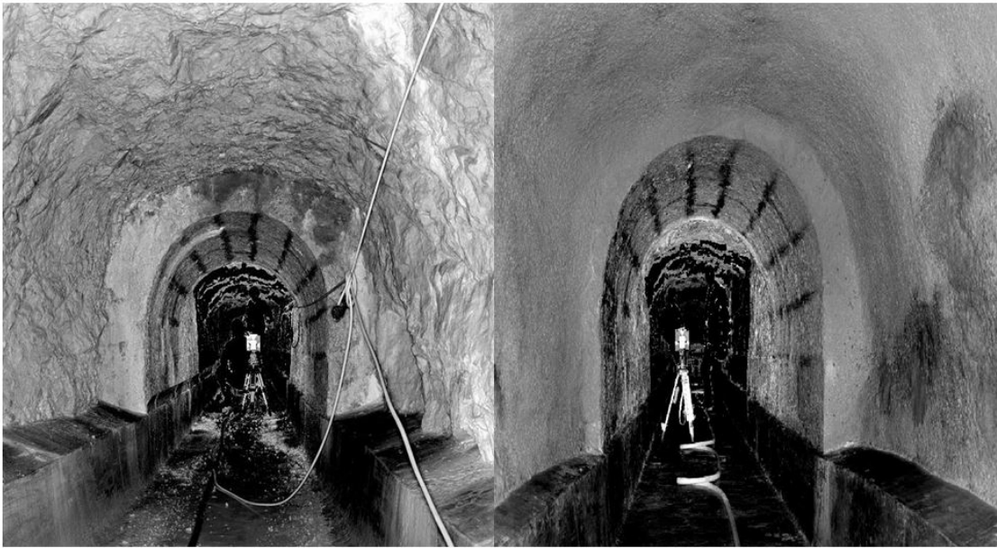
Fig.6 – Water transfer tunnel (Copyright: Stadt Wien)
