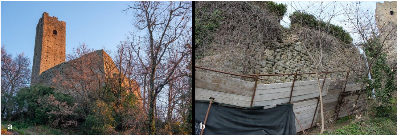
Fig. 1. The fortress of Larciano (a), and part of the eastern wall (b). Vegetation, collapses, safety precautions and the steepness of the ground are visible.
