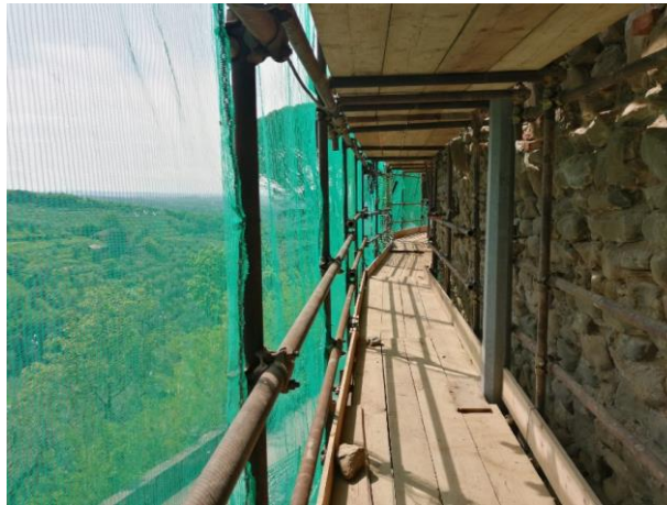
Fig. 2. The scaffolding of the wall: the floors made hard to obtain vertical overlap and it forced to take very close images
