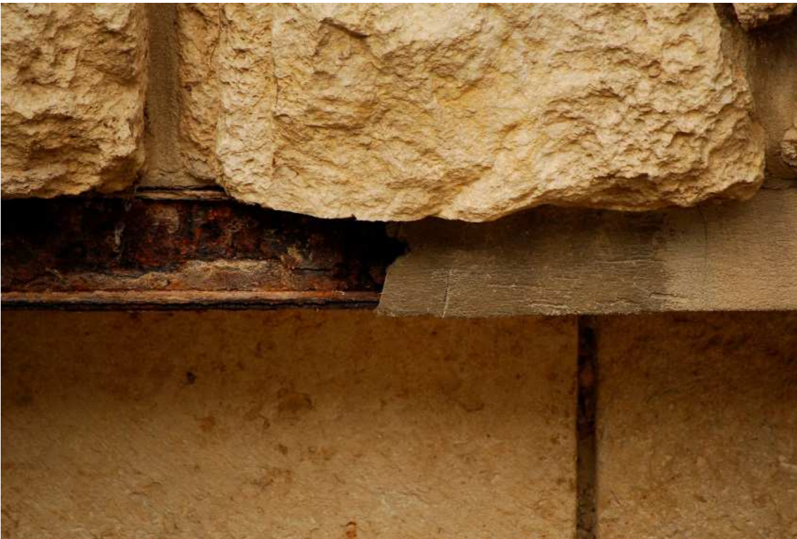
Fig. 11 – Ejecting the concrete cover in the beam on the foundation of the aisle facing north.
