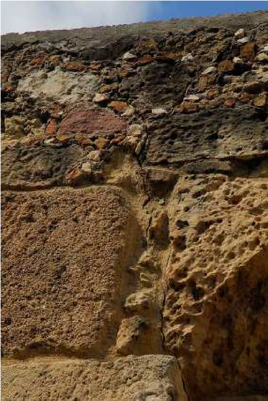
Fig.8 – Cracks along the Aisle facing south.
