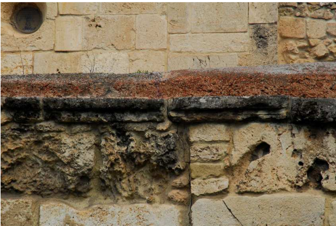
Fig. 7 – Cracks along the Aisle facing South.
